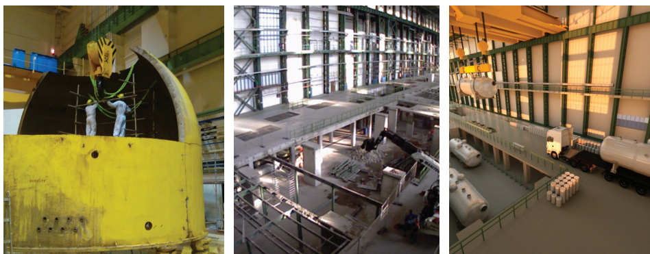
Above (from left to right): Fragmentation of one of the reactor shaft protection lids
