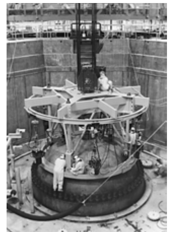
U.S. plant outage showing six TENSOR™ tensioners, a rigid pole system and head lift rig/carousel
