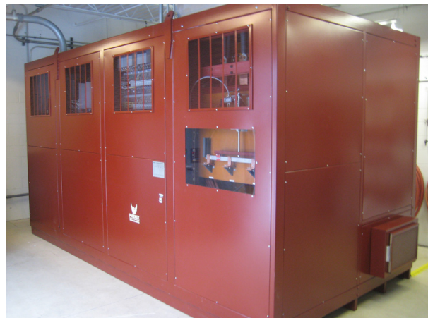
Main power cabinet
