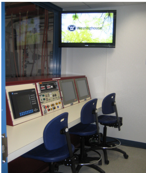
State-of-the-art control room
