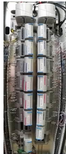
Ovation Cabinet Front Interior
