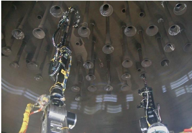
Gemini system performing NDE on two RVH penetrations in parallel (J-Groove weld UT and Thermal Sleeve Thickness UT)
