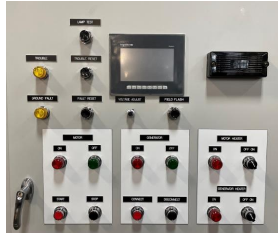
Typical Next Gen Cabinet Front
