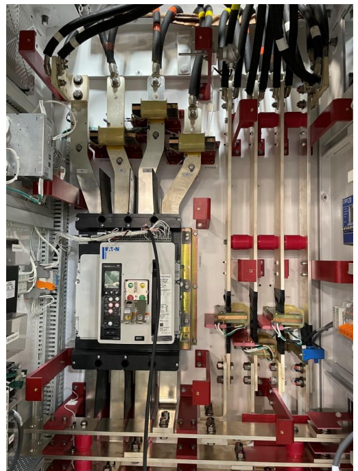
Internal Cabinet Backpanel with safety shields removed
