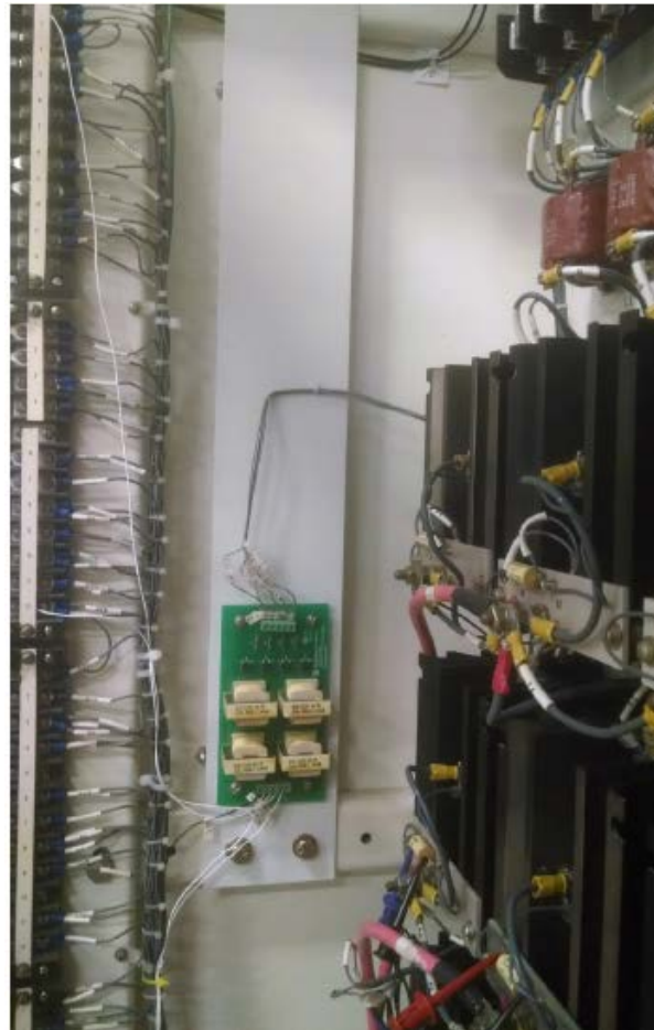
Loss of 120 VAC Modification Installed in Power Cabinet
