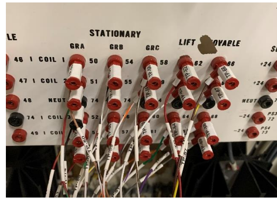
Custom Cabling Included to Interface with A70 Test Panels in Power Cabinets
