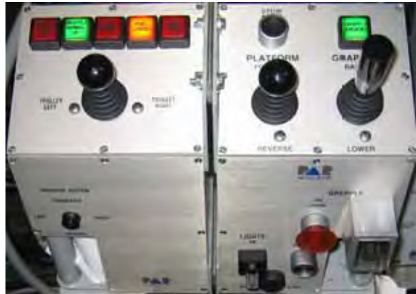
BWR replacement controllers
