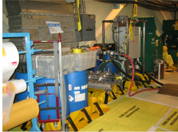
Typical inside TTS ASCA/CODE equipment setup
