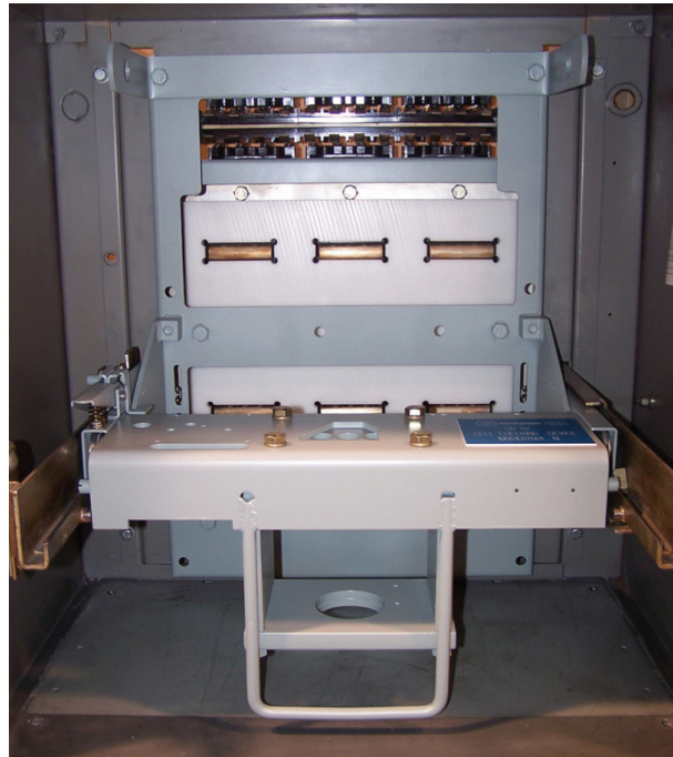
DB-50 cell checking device installed in cell
