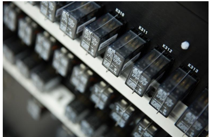
Maintenance Enhanced Relay Mounting
