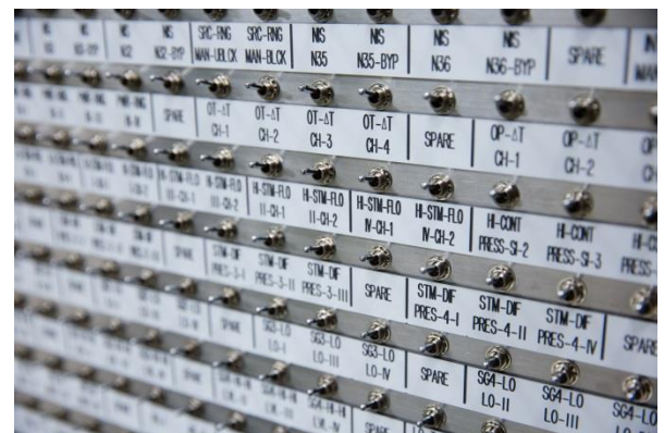
Switch Test Panel
